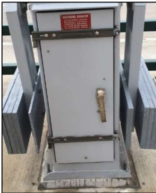
Figure 3: Control cabinet door with crossbars
