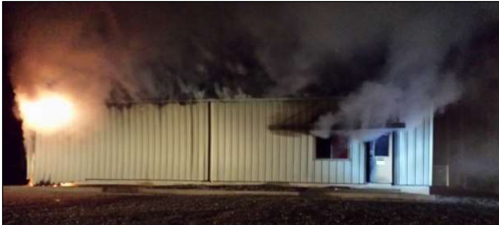
Figure 7: Sabotaged substation control house
