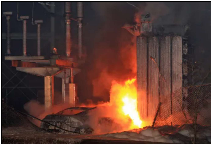
Figure 8: Automobile crash with transformer fire in 138 KV substation
